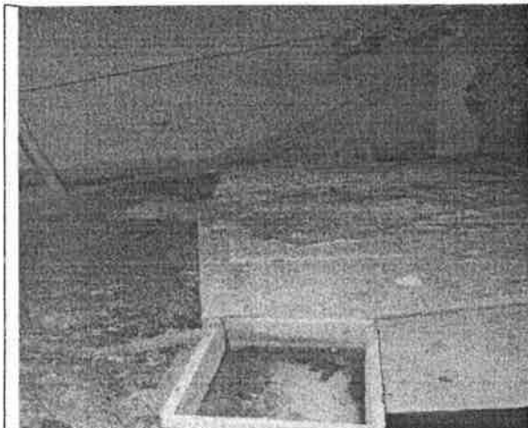
leakages are stagnated in the drain of industry premises;
