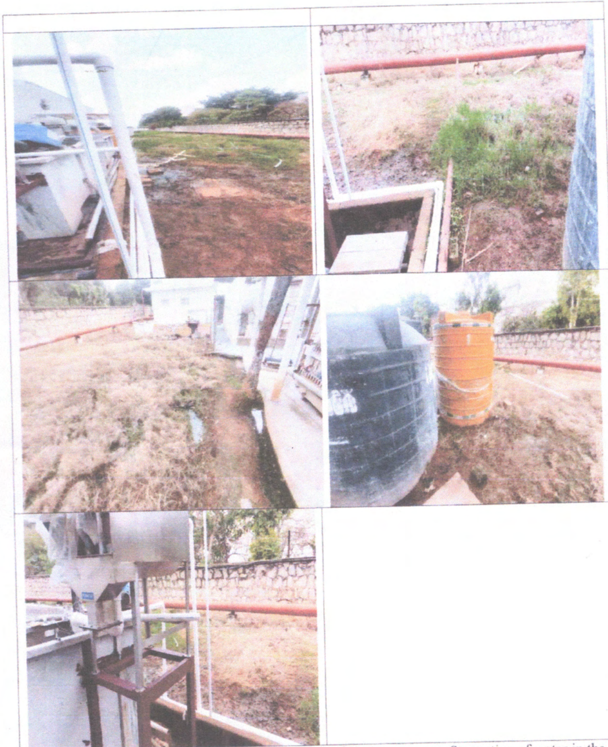
Treatment facility area and its back area – housekeeping is very poor. Stagnation of water in the back side of the treatment plant and algal growth formation
